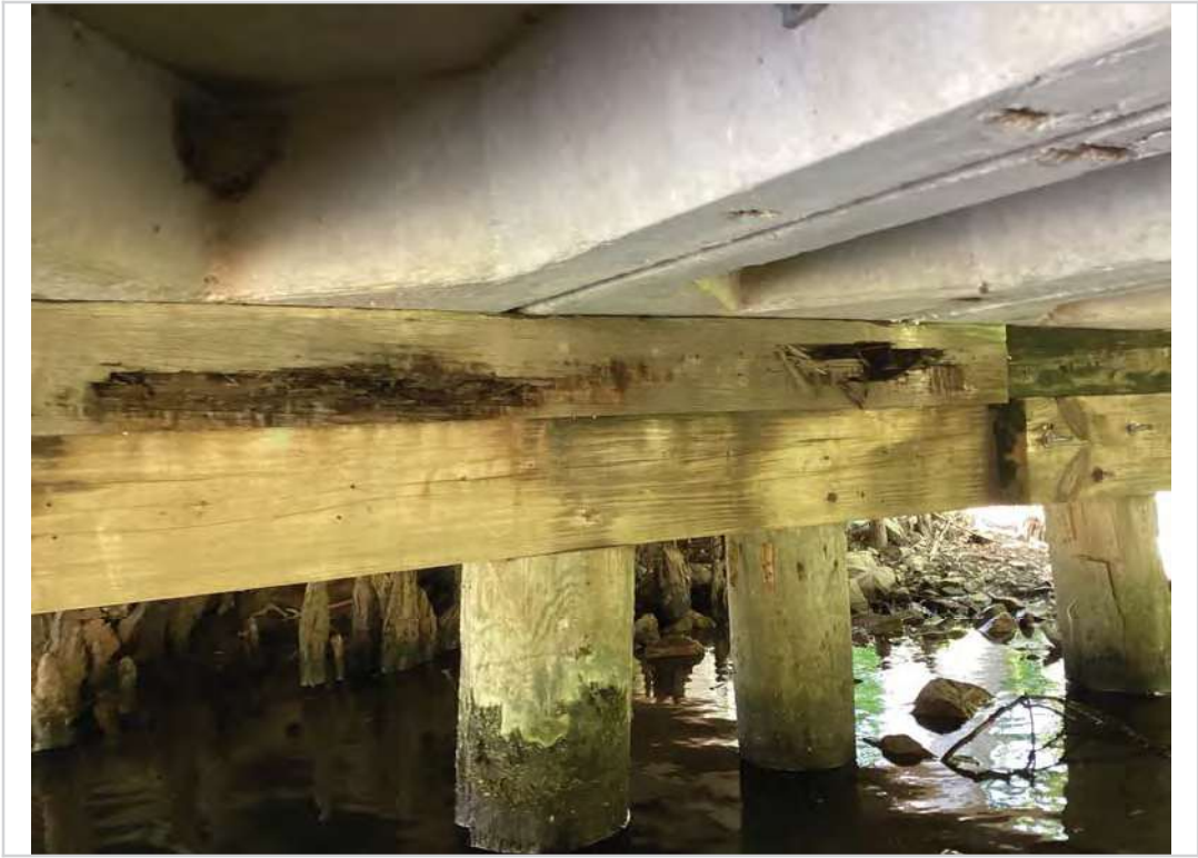
Decay areas bent 1 rear
